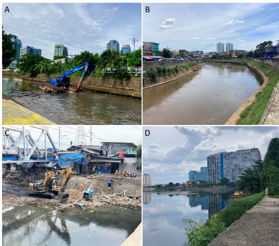
Figure 10: Flood protection measures in Jakarta, A-River dredging at the Ciliwung, B-River canalization of the Ciliwung, C-Rebuilding embankments at the Kali Krukut River, D-Pluit Reservoir
