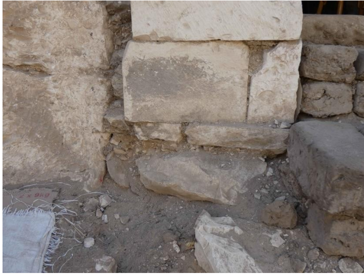
Pl.7. The frontal view of the reparation of the eastern doorjamb with limestone block.
