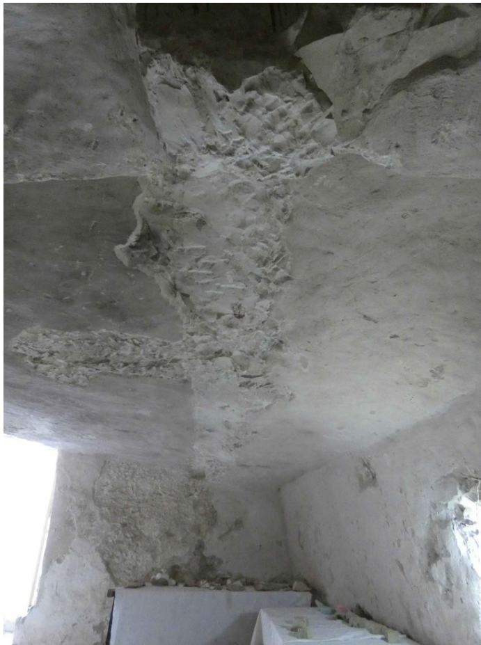
Pl. 122. Details of a badly chiseled off architrave.
