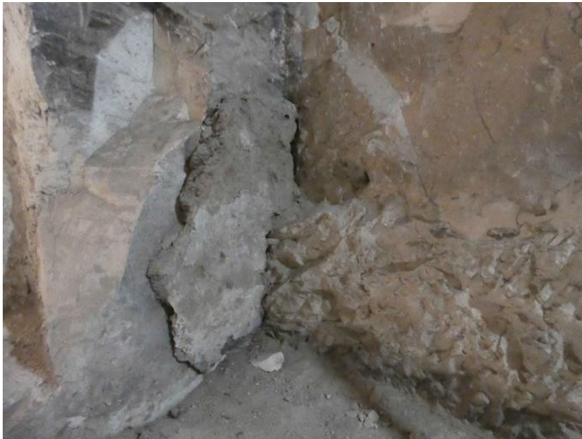
Pl. 34. Plaster remains in the north-east corner.
