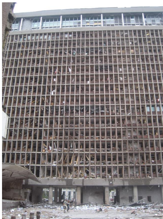
Figure 1 - The building housing the Office of the Prime Minister and Ministry of Justice and the Police with blown-out windows shortly after the explosion. The bomb van had been placed behind the people shown.[1]
